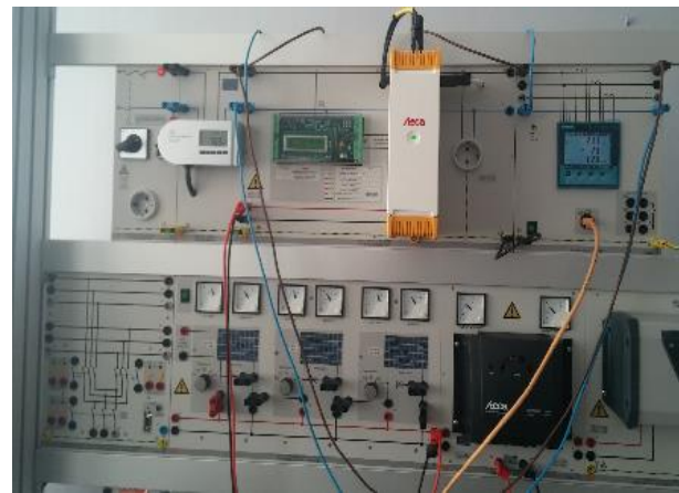
Figure 13. Lab setting for the Experiment: Photovoltaic system with On-grid inverter.
